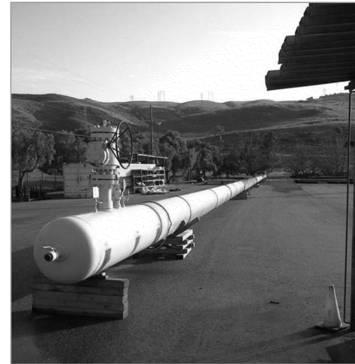
Testing equipment, such as above ground pipes and valves
