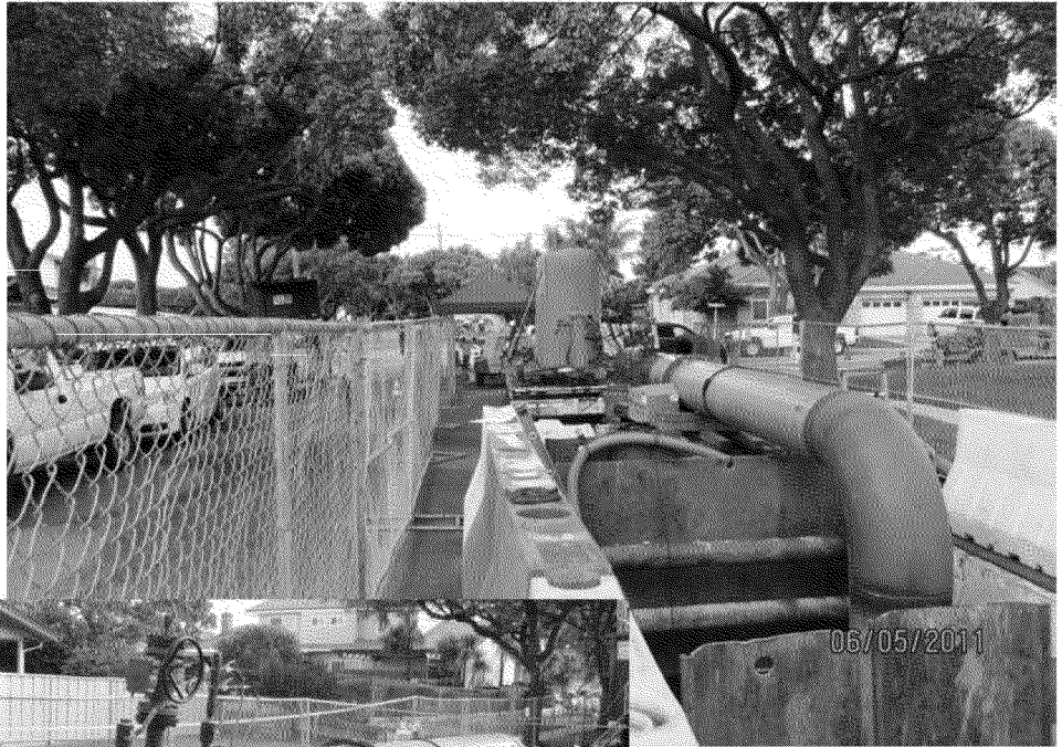
Test Header and Above Grade Piping
