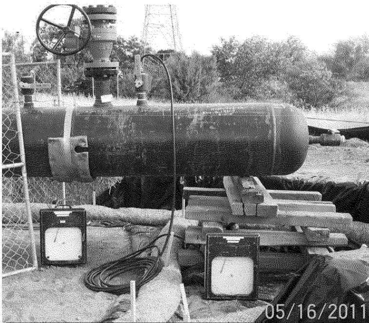
Test head and pressure monitoring valve header used to monitor test segment pressure
