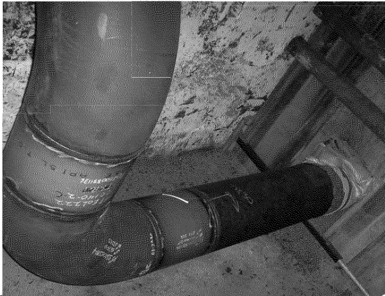
Exposed Test Segment piping
