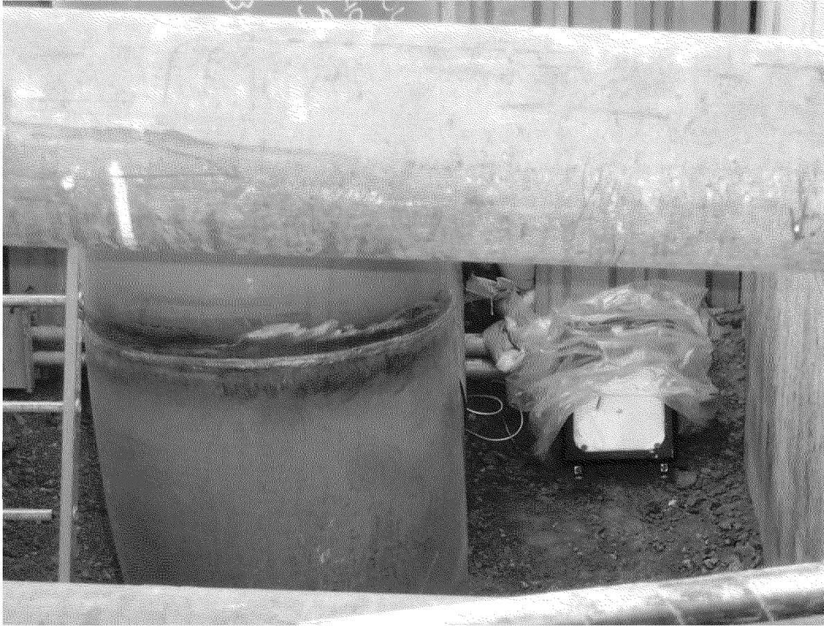
Restrained Pipe temperature monitoring installation and chart recorder
