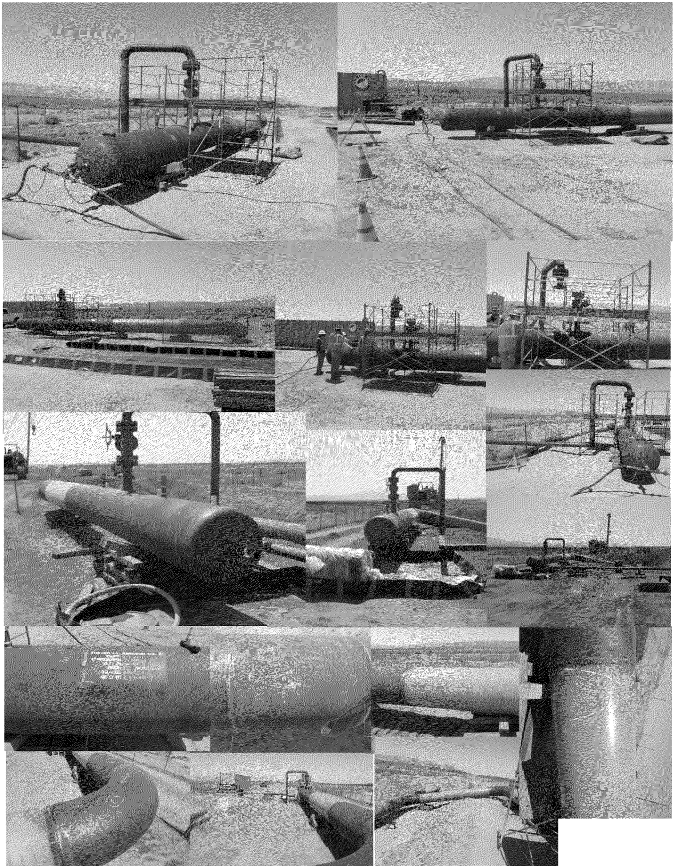
Exposed Test Headers and Piping
