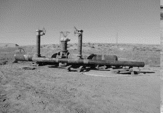
T-62 Block Valve Cutout
