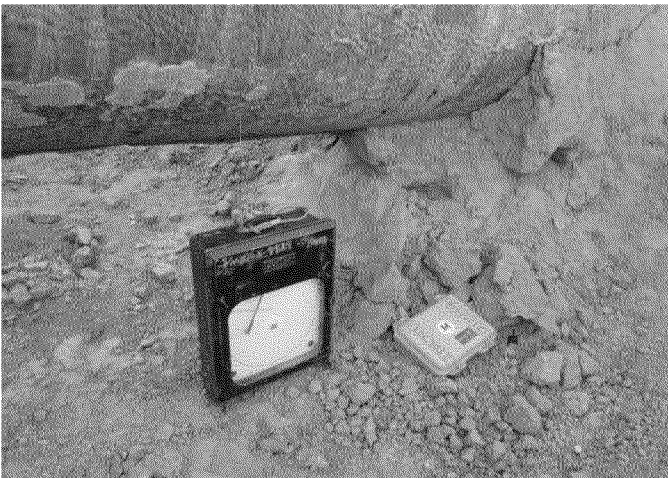
temp. recorder on restrained pipe at location A test 85
