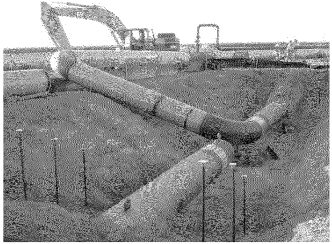
test head piping at location A, test 85
