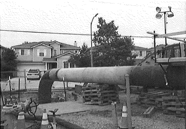
Test Header at Location A
