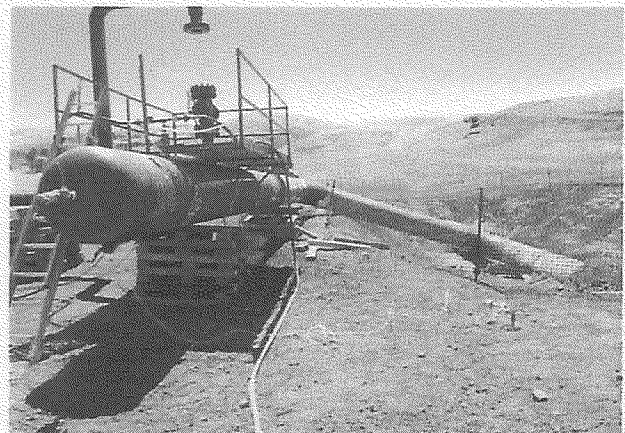
Test 89S testhead at location E
