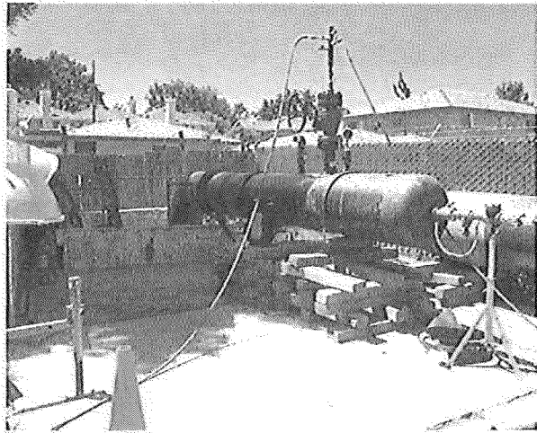
Test Header at location A
