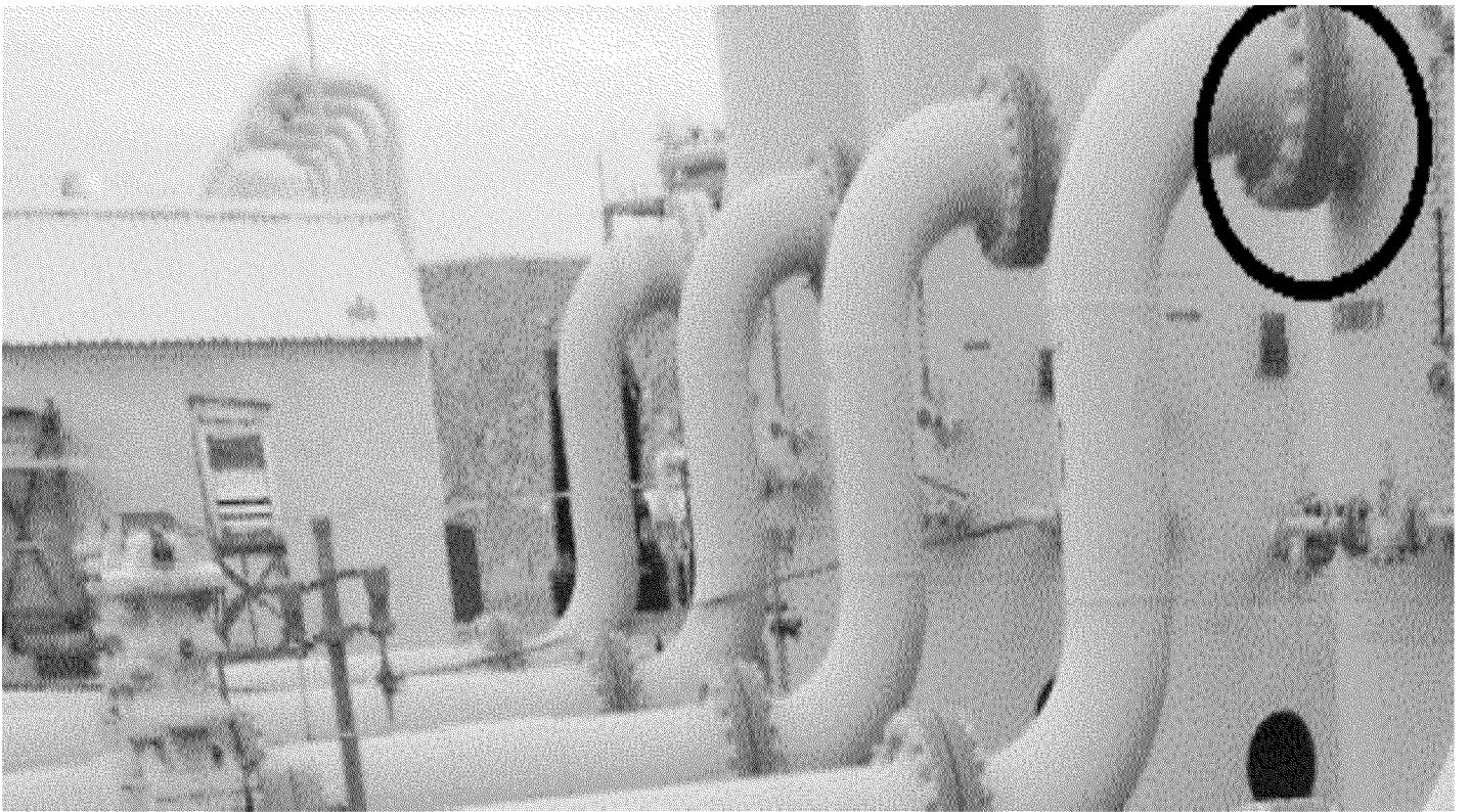
Photo #5 – 3A Scrubber line 16” flanged connection
