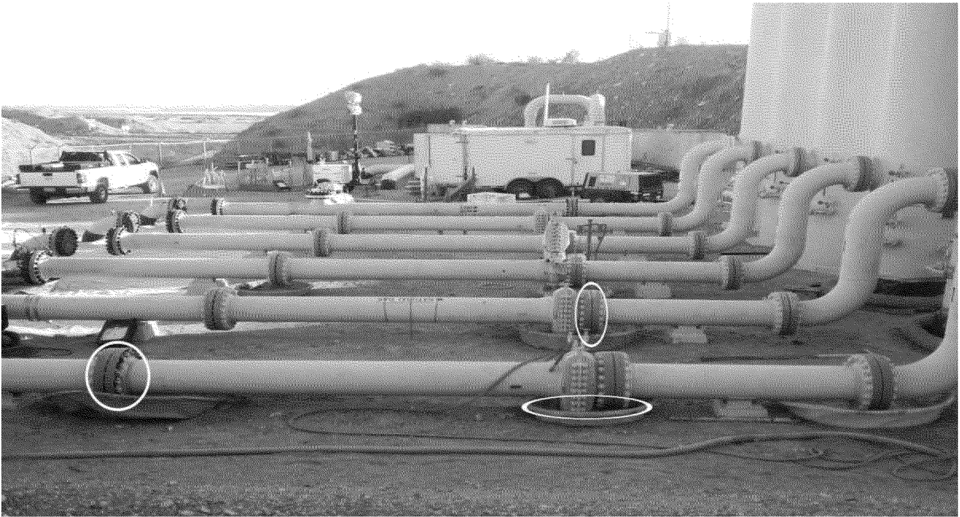
Photo #13 – 1B and 2B Scrubber lines flanged connections and orifice meter
