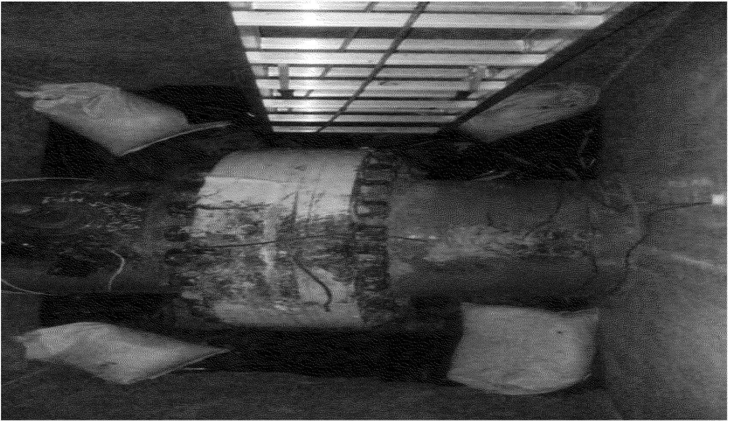
Photo #11 – B1 valve insulating flange
