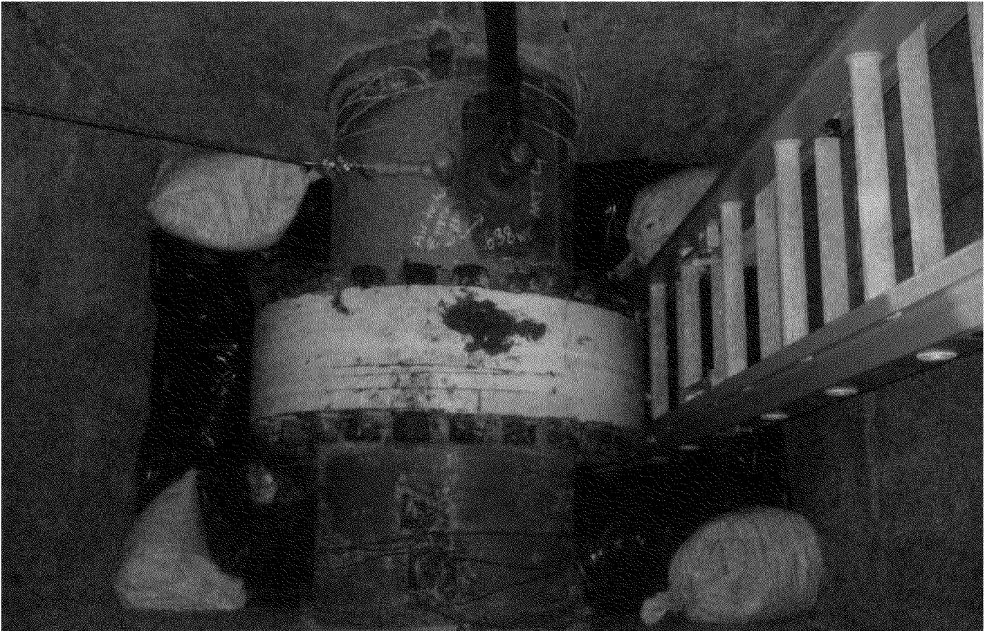
Photo #12 – B3 valve insulating flange
