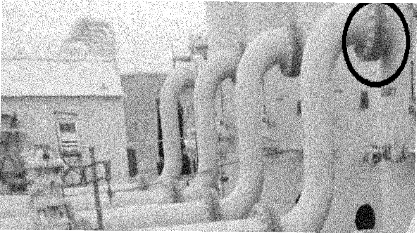
Photo #5 – 3A Scrubber line 16” flanged connection
