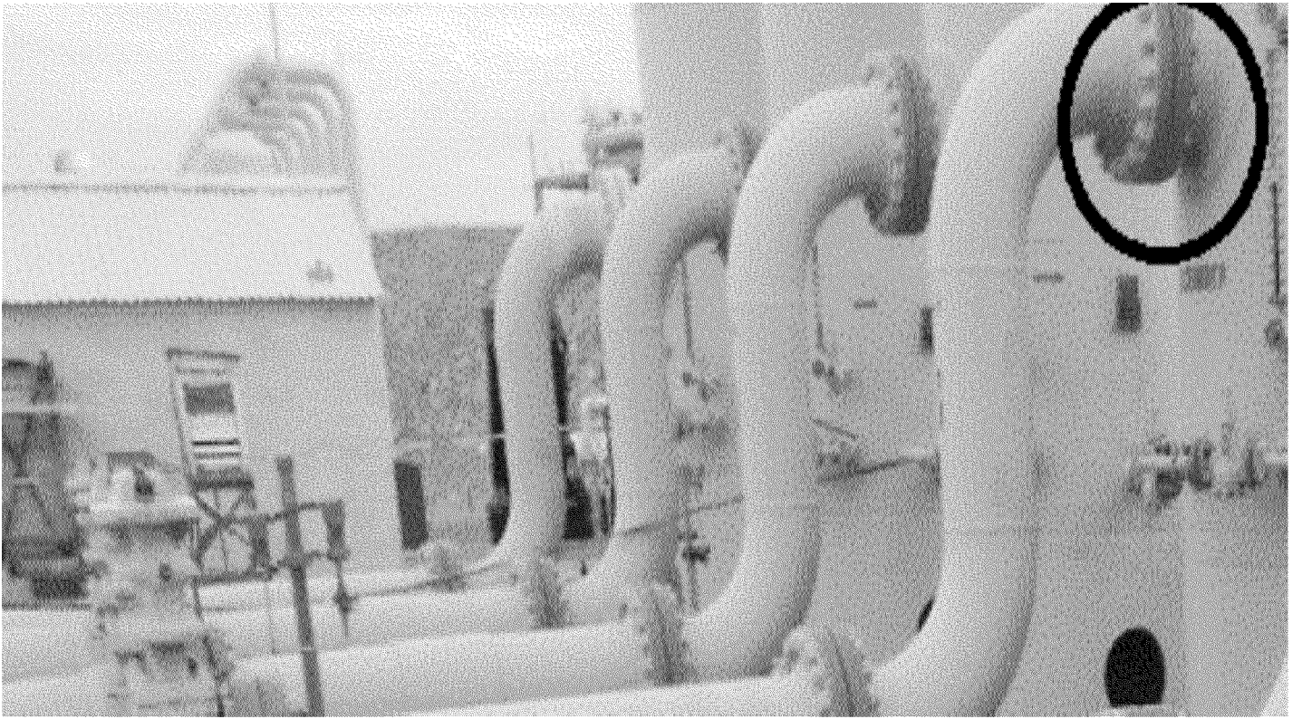
Photo #5 – 3A Scrubber line 16” flanged connection
