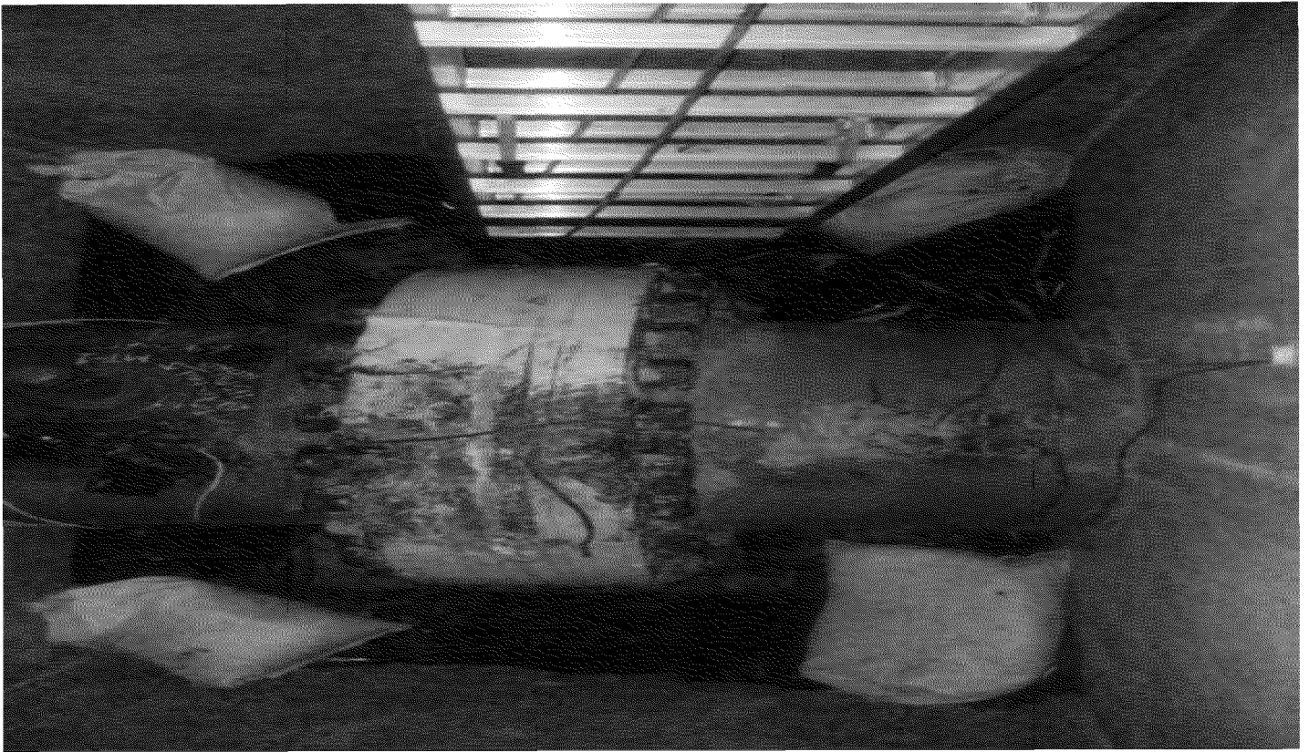
Photo #11 – B1 valve insulating flange
