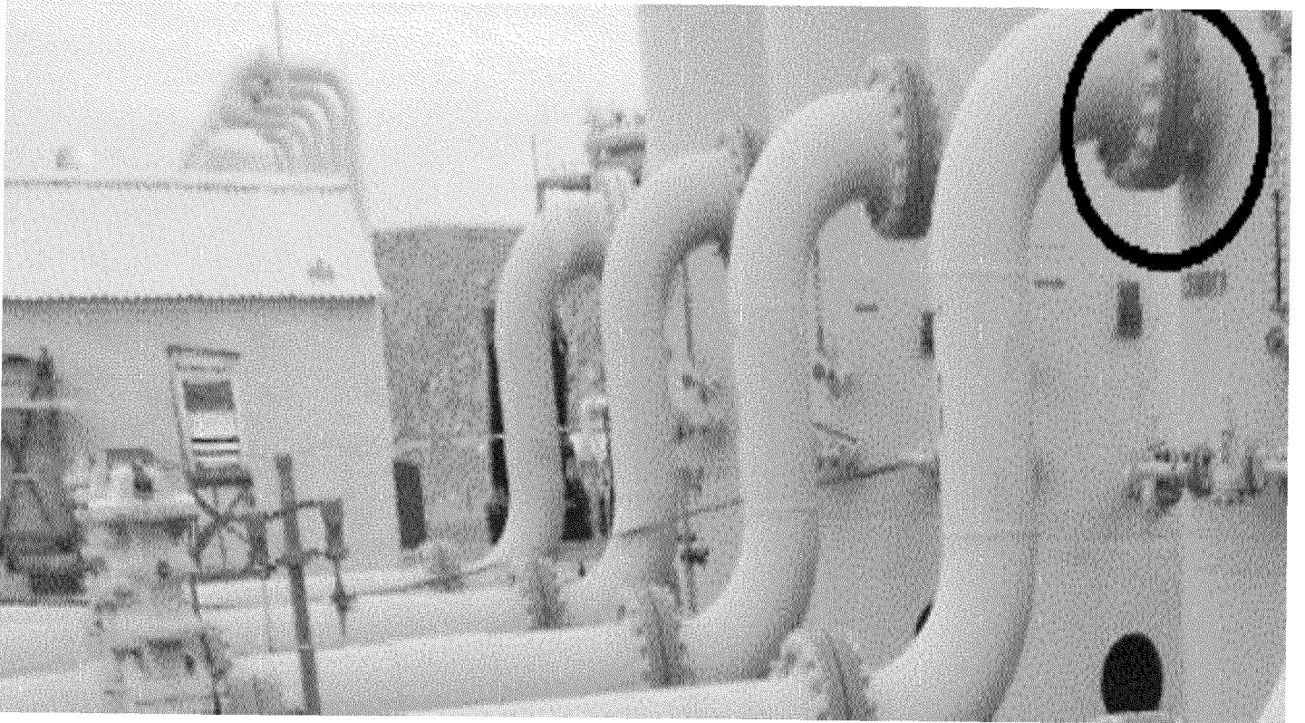
Photo #5 – 3A Scrubber line 16" flanged connection
