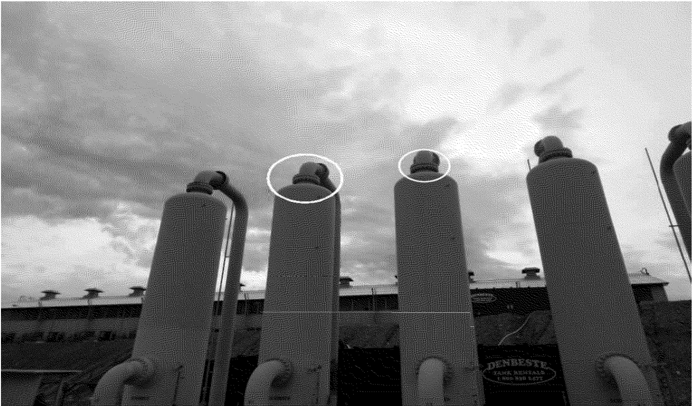
Photo #8 – 4A and 5A Scrubber lines 16" flanged connections
