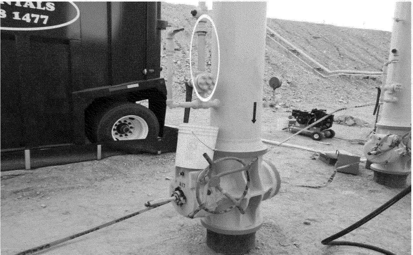
Photo #4 – 3A Scrubber line relief valve union
