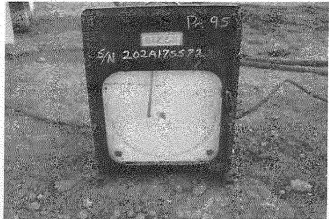
Test T-65A Pressure Gauge
