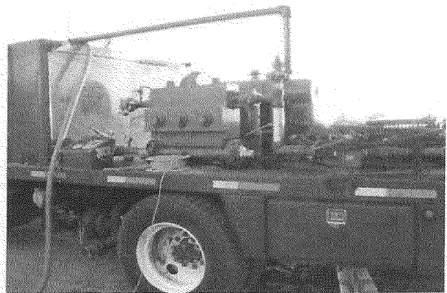
Test T-65A Pump truck
