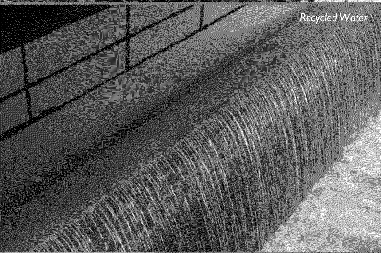
San Jose Creek Water Reclamation Plant
