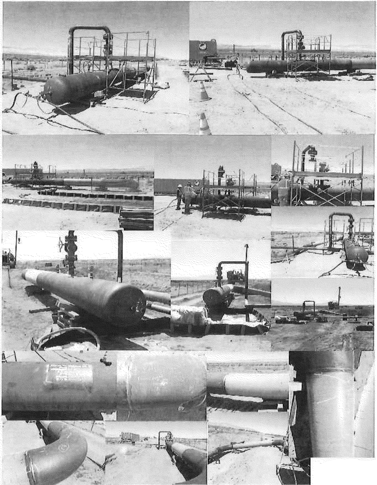
Exposed Test Headers and Piping
