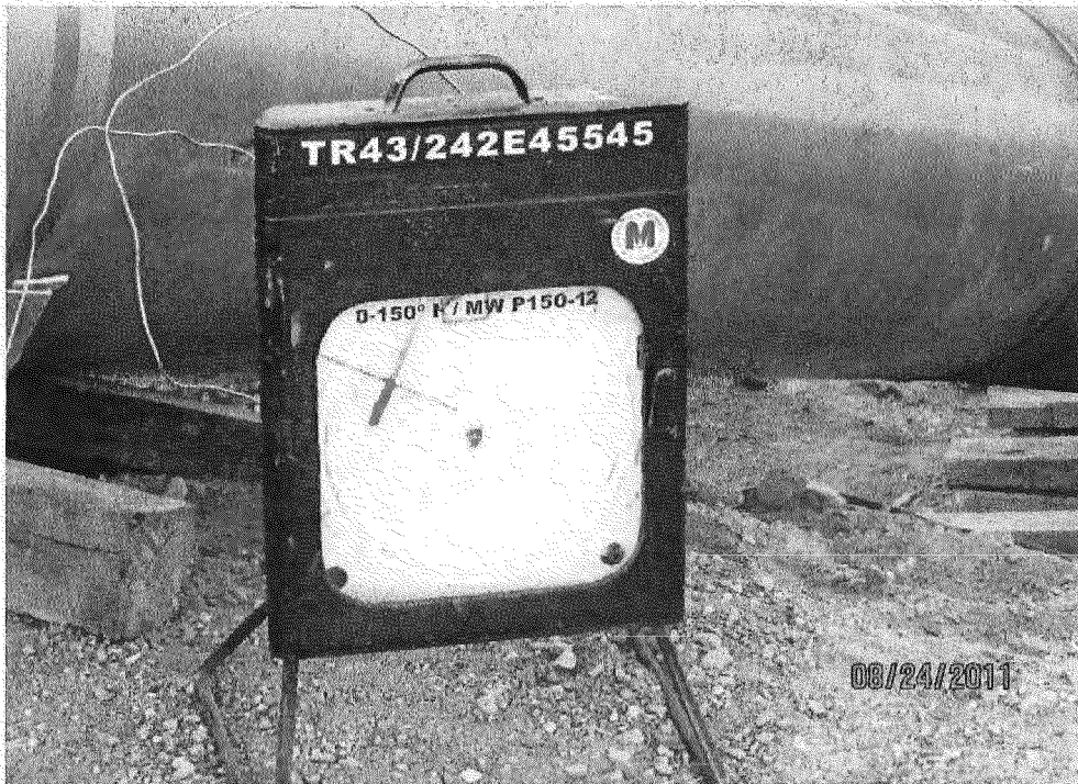
Unrestrained Pipe Temperature Recording Chart
