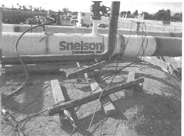
Test Head Cross over piping
