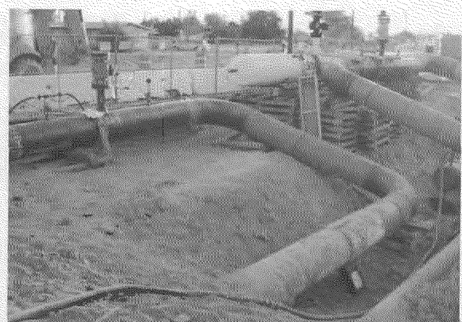
test 75 Location B dual temp recorder restrained and unrestrained pipe temp.
