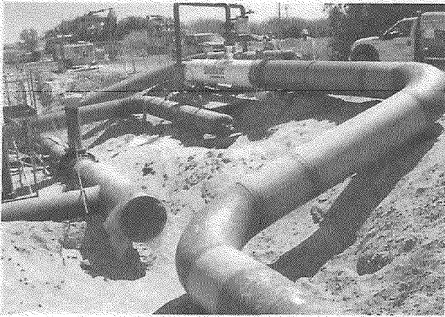
test 56 Loc.B test head in white on 34"mainline
