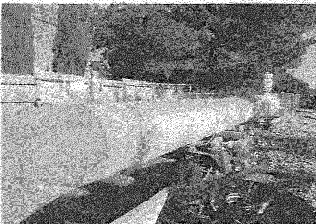
Test 34 Loc. A riser and test head
