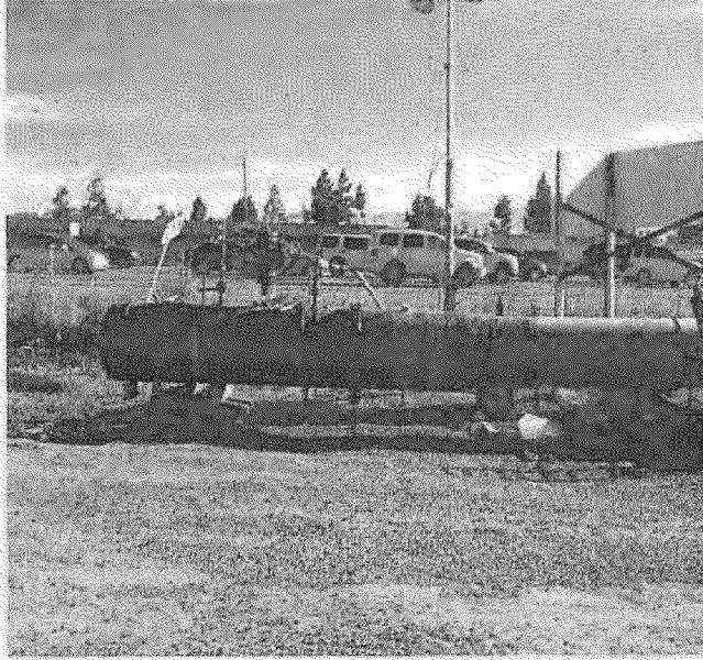
North Segment Test Header
