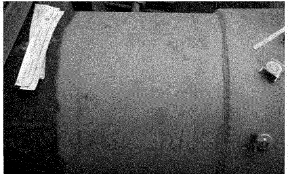
Overview of Ext. Metal Loss and Pitting
