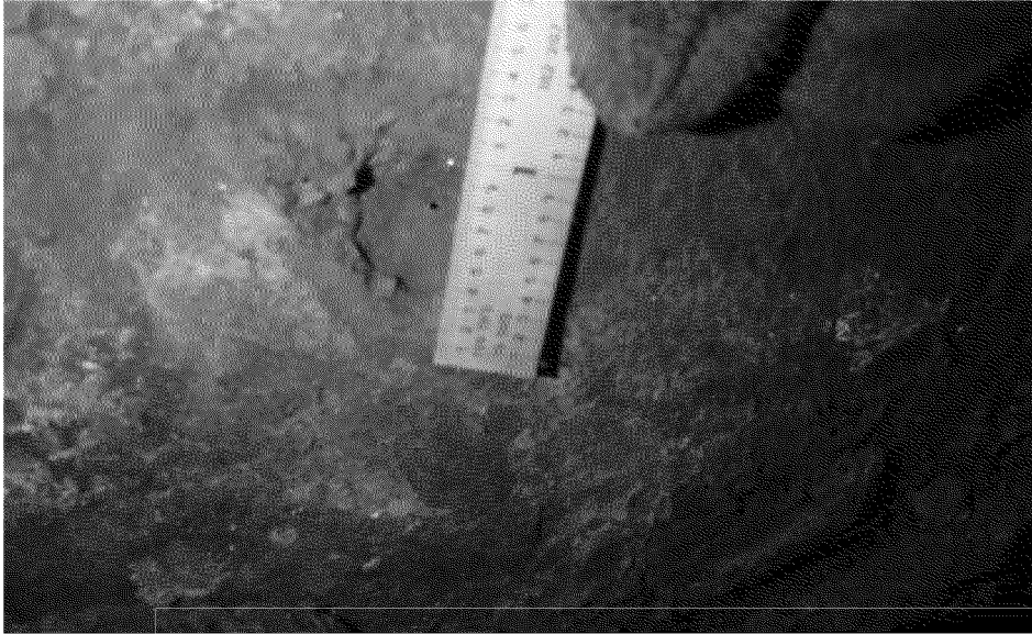
Close up of leak
