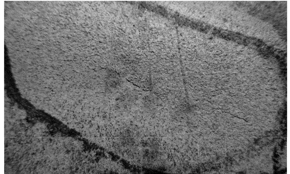
Close up of second inspection MT Indications of LIN-07
