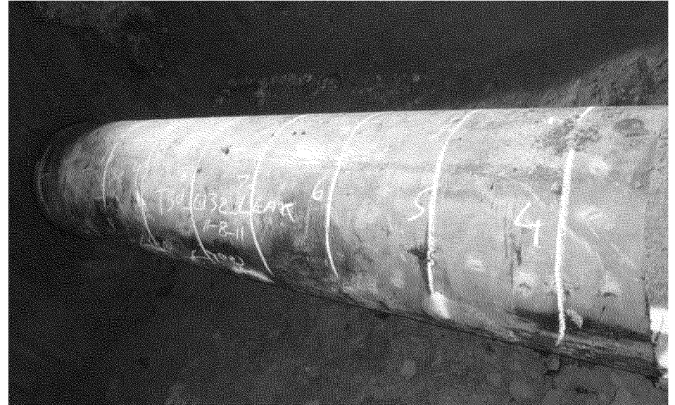
Overview of deposits layout 3.50ft to 12.35ft, 9:00 position
