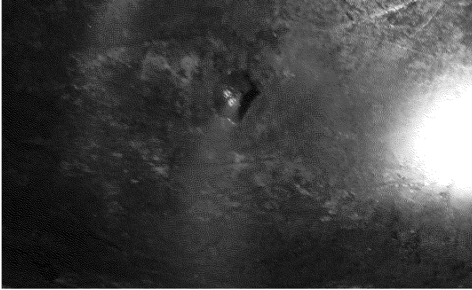
Close up of DEP-01
