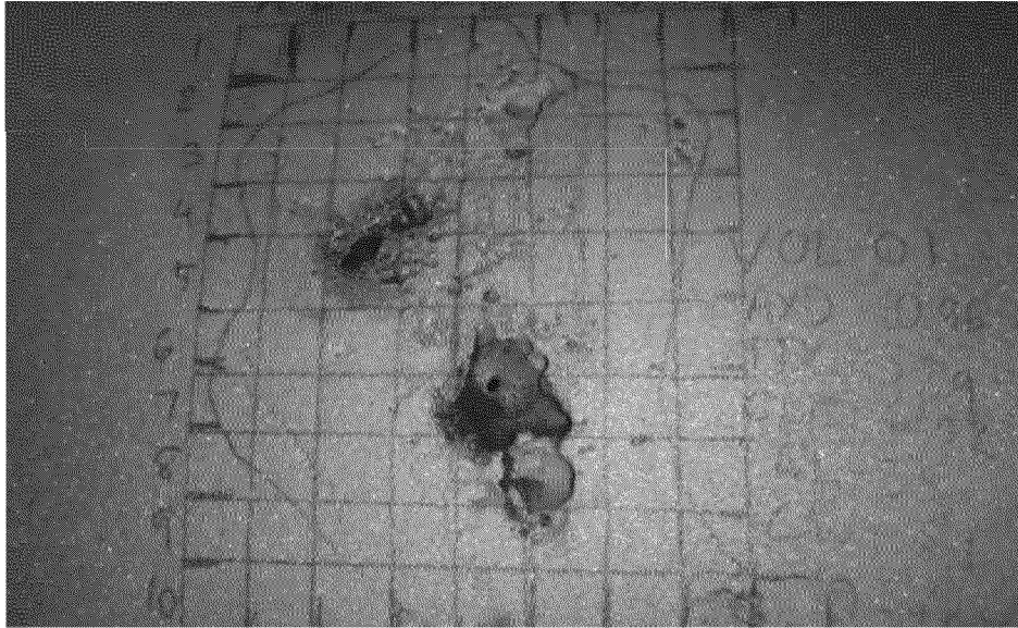
Overview of corrosion grid VOL-01
