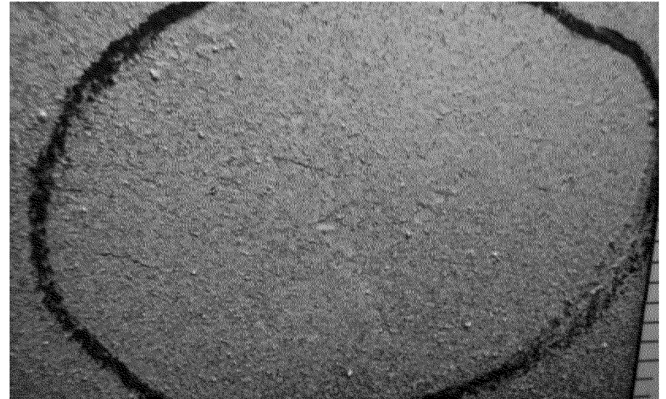
Close up of second inspection MT Indications of LIN-03
