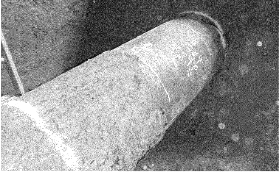
Overview of coating condition 8.00ft to 13.00ft, 3:00 position
