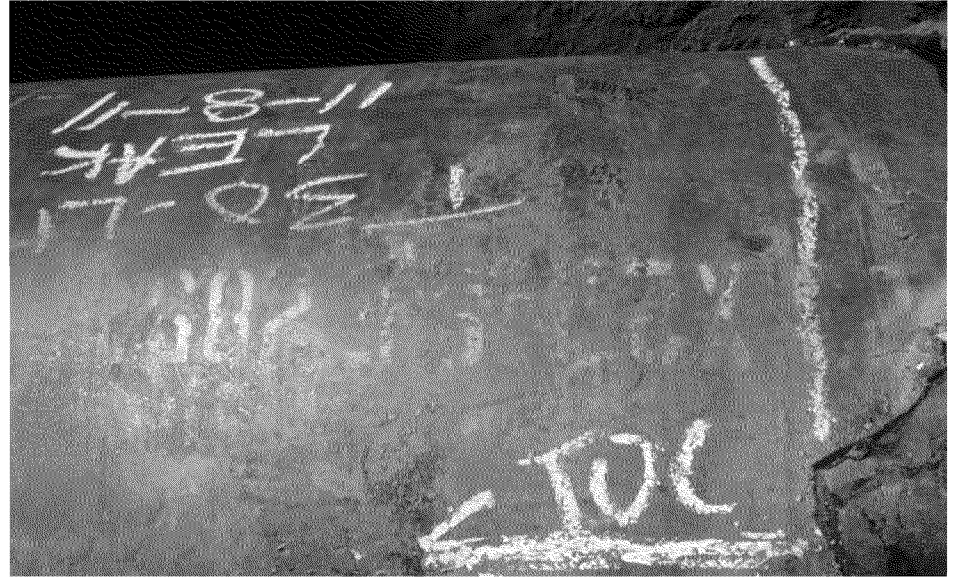
Close up of pipe stenciling
