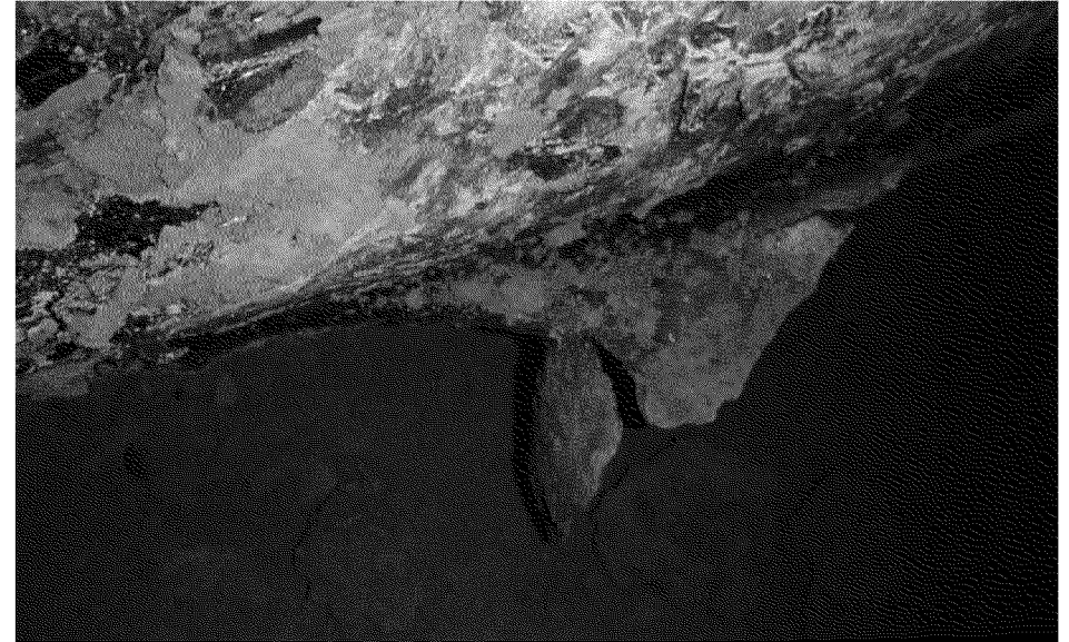
Close up of DIS-01 and coating removed to find leak
