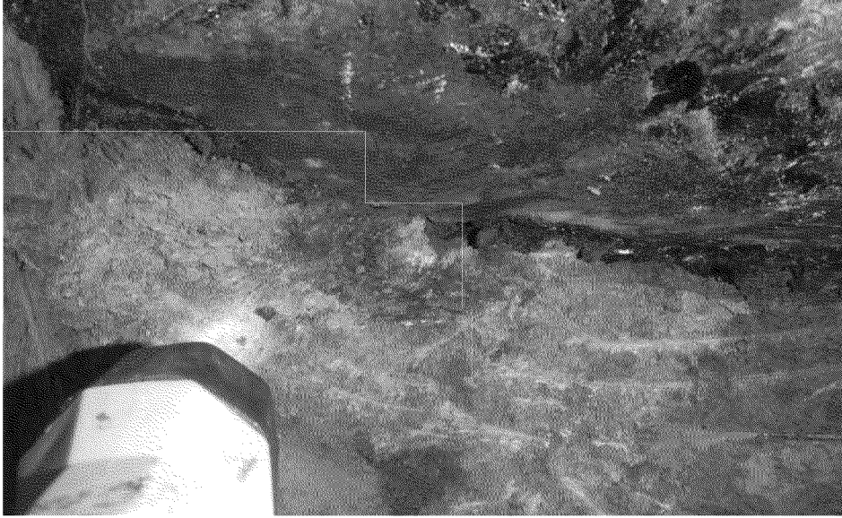
Close up of leak
