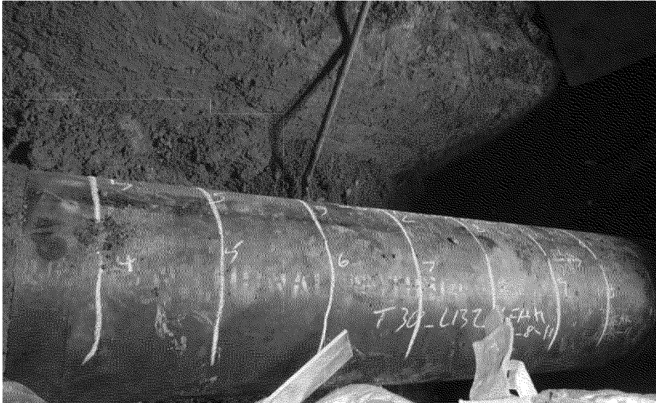
Overview of deposits layout 3.50ft to 12.35ft, 3:00 position
