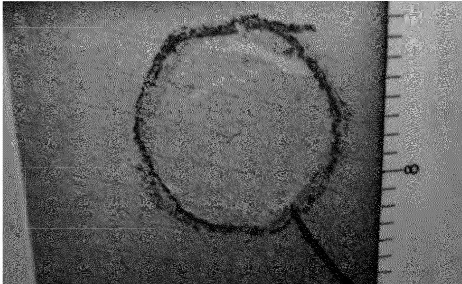
Close up of second inspection MT Indications of LIN-18
