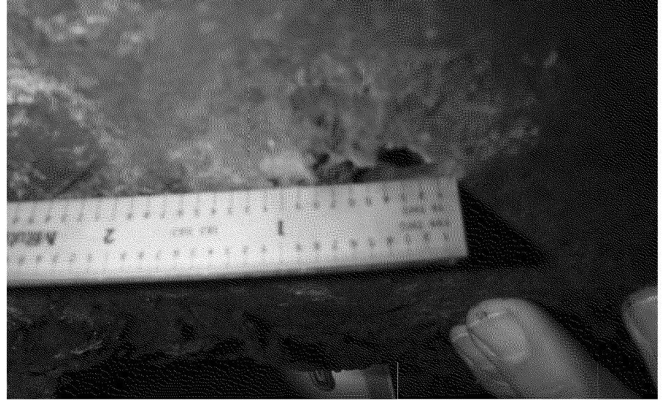
Close up of leak
