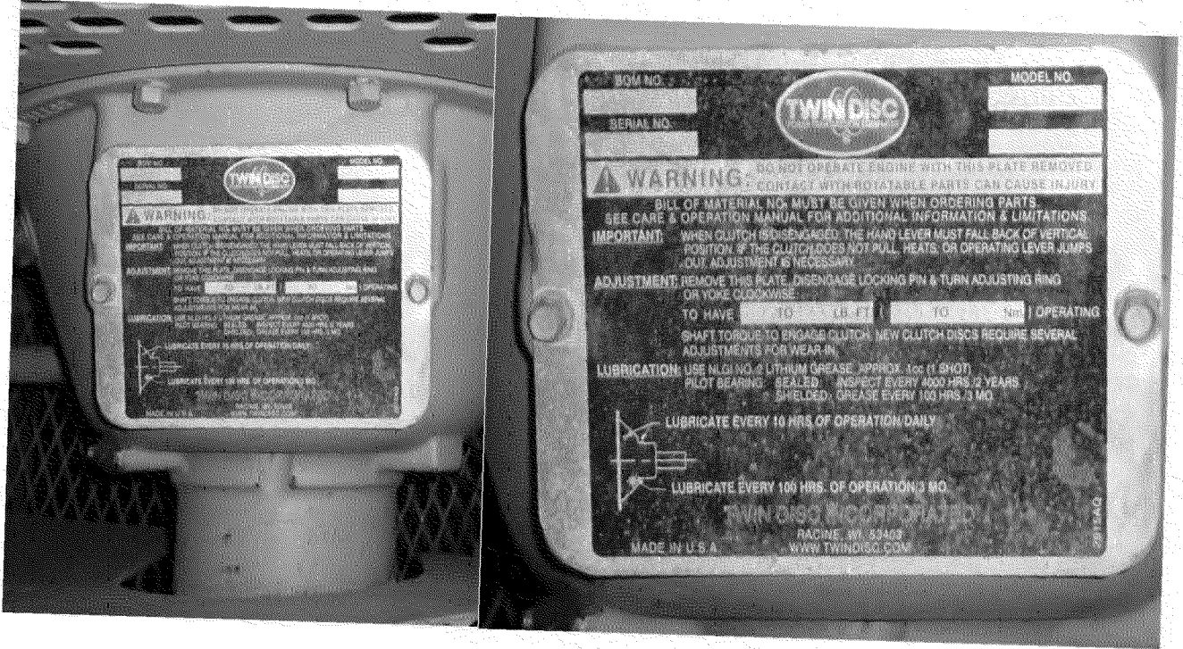
Test Pump Name Plate
