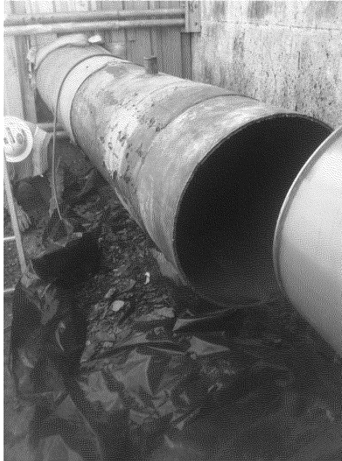
5 6 7 8 9 10 11 12 13 14 15 16 17 18 19 20 21 Illustration C: Coating Deficiencies
