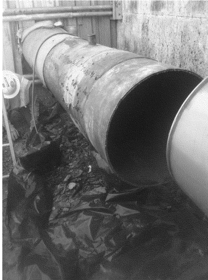
5 6 7 8 9 10 11 12 13 14 15 16 17 18 19 20 21 Illustration C: Coating Deficiencies
