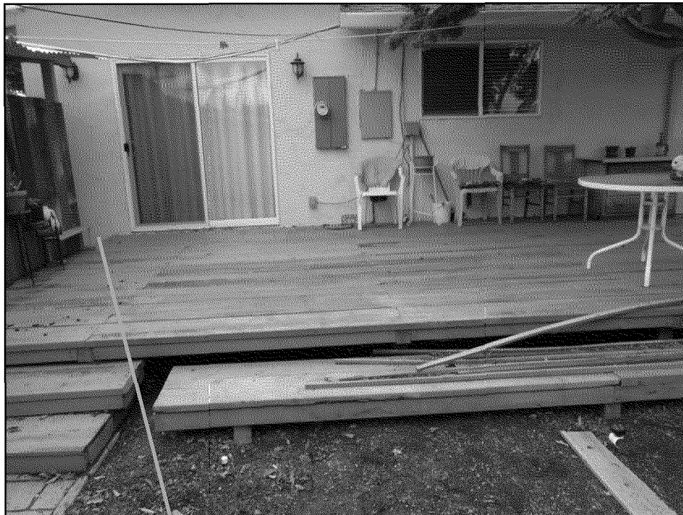
Deck is over the top of the line.
