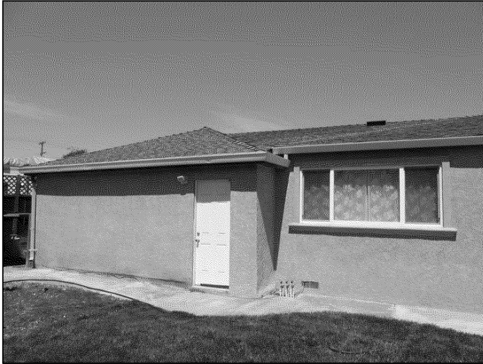
1.43' of the house is within the easement area.
