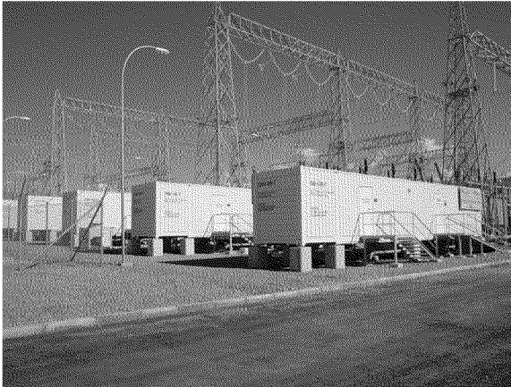
Figure 1: View of the BESS installation in Northern Chile
