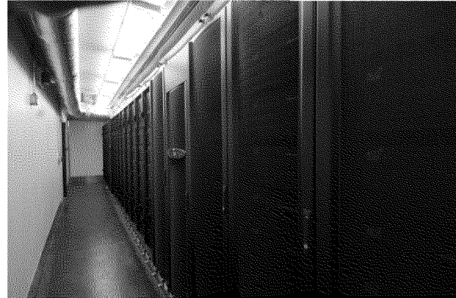
Figure 2: View inside a BESS container
