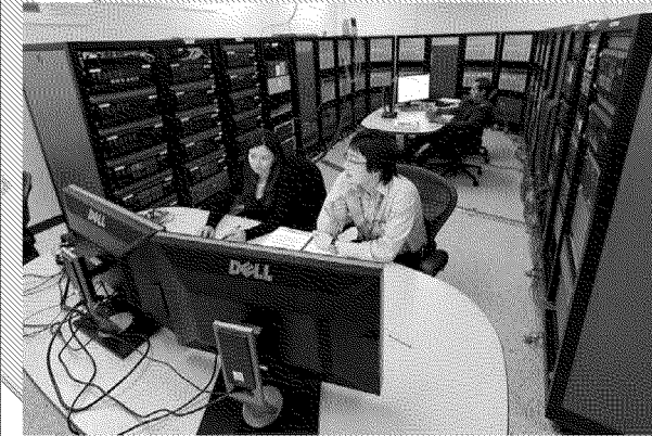
RTDS Lab at Southern California Edison
