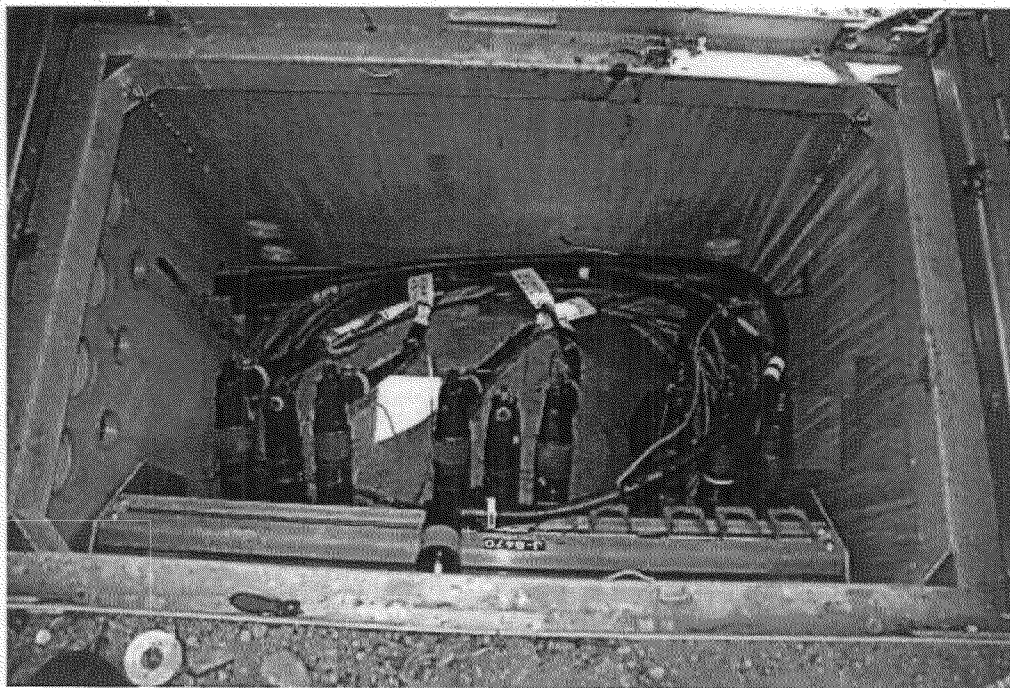
Picture 1 Junction Box
