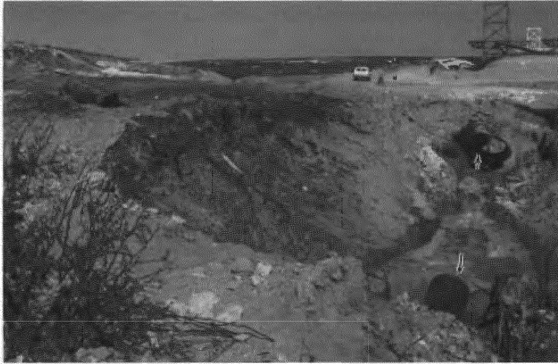
Figure 6. Looking west at a portion of the crater created by the rupture. The missing section of pipe between the arrows was ejected from the crater.
