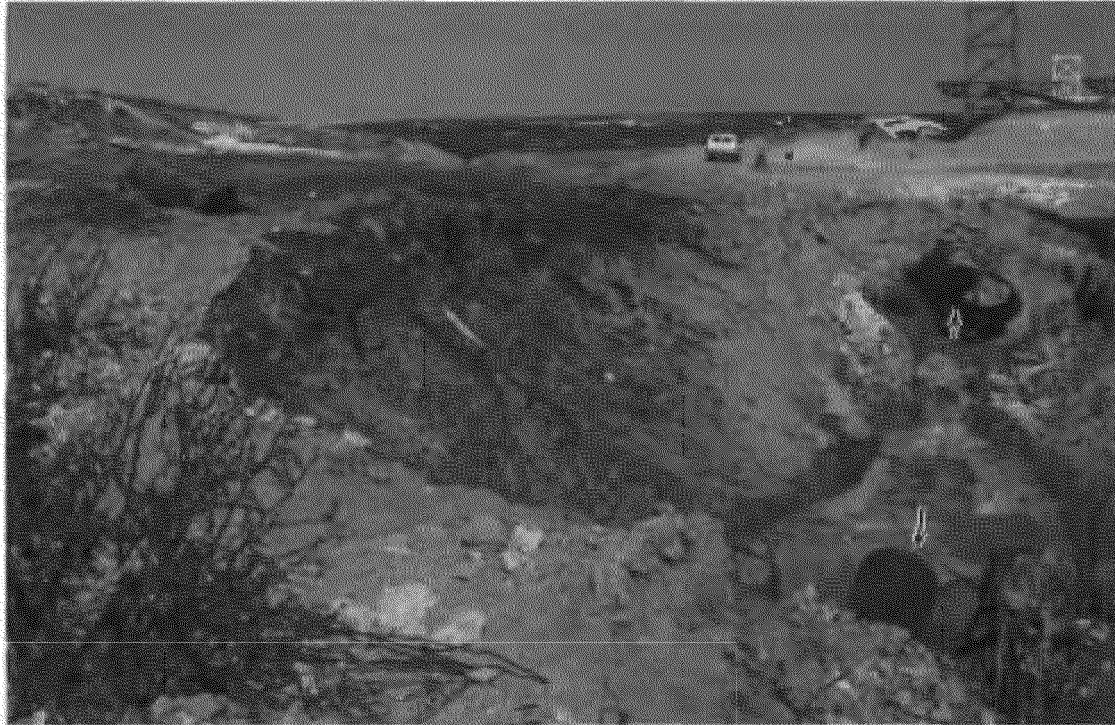
Figure 6. Looking west at a portion of the crater created by the rupture. The missing section of pipe between the arrows was ejected from the crater.
