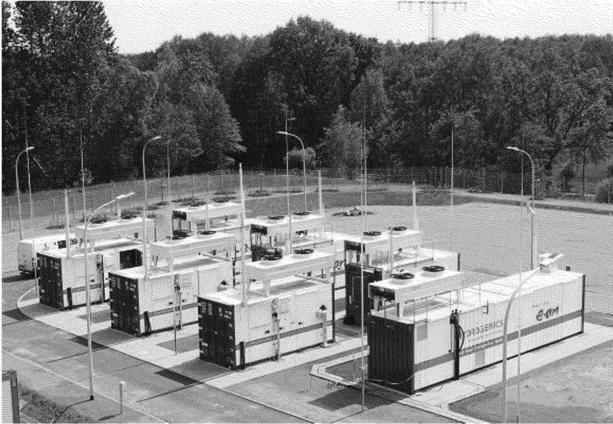
Exhibit 5 – Operating Hydrogen Energy Storage (Power-to-Gas) Facility in Falkenhagen, Germany
