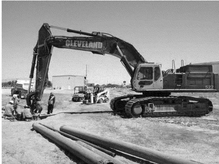
Photo 13. Removed pump casing and driveshaft from WS1. Attempting to free remaining pump from the well. Looking east. April 18, 2013.
