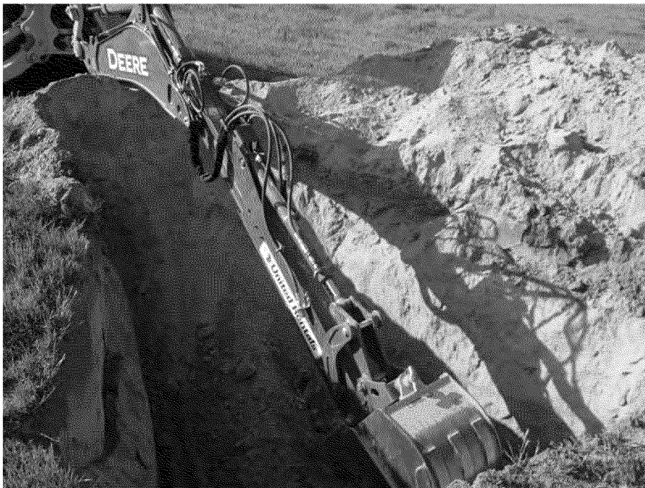
Photo 6. Reaching final depth of approximately 8 feet below ground surface in location 1. Looking northwest. March 12, 2013.
