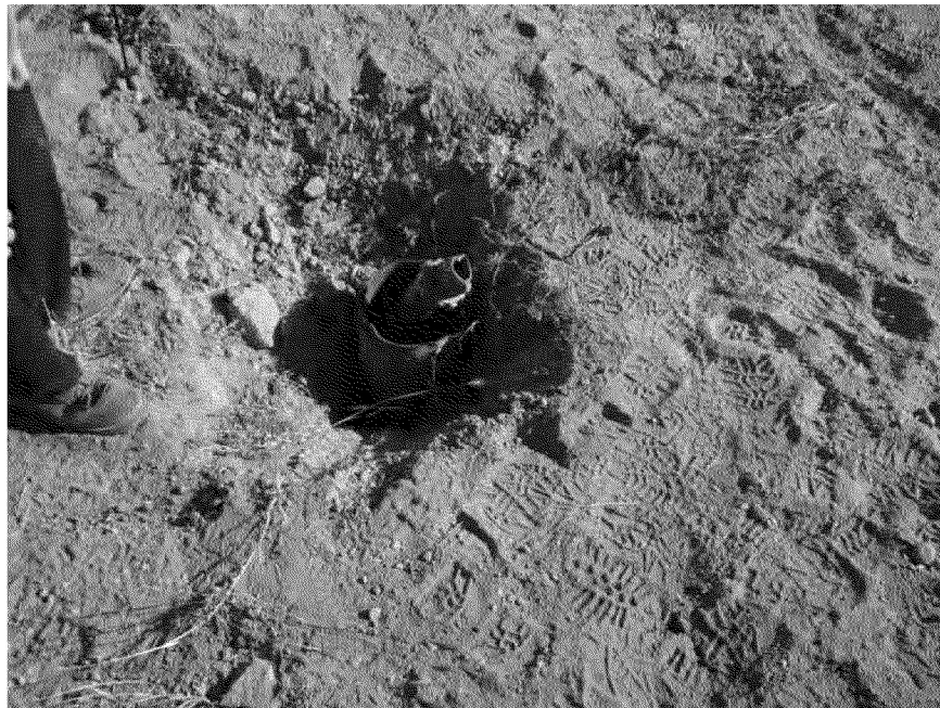
Photo 9. WS1 prior to pump removal attempt. Visible is the 10-inch diameter pump casing and interior oil tube/driveshaft. Looking north. April 16, 2013.
