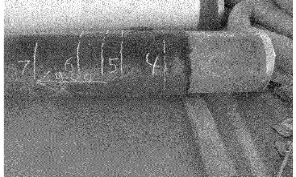
Overview of coating condition 9:00 position
