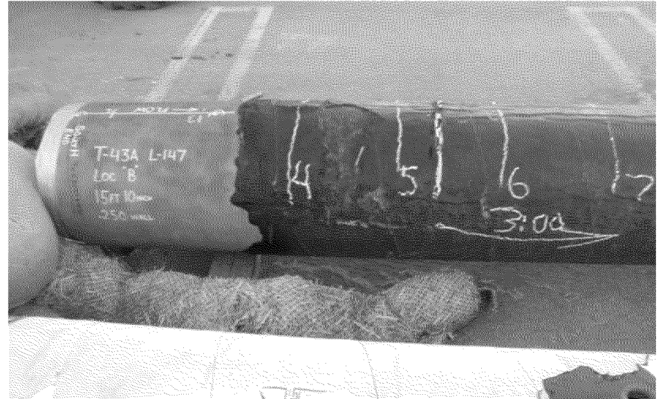
Overview of coating condition 3:00 position
