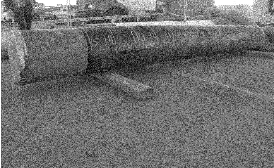
Removed pipe section coating assesment 9:00
