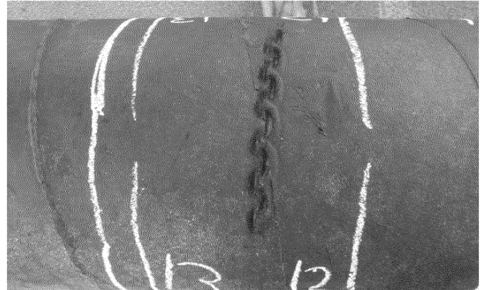
Coating damaged from removal process.
