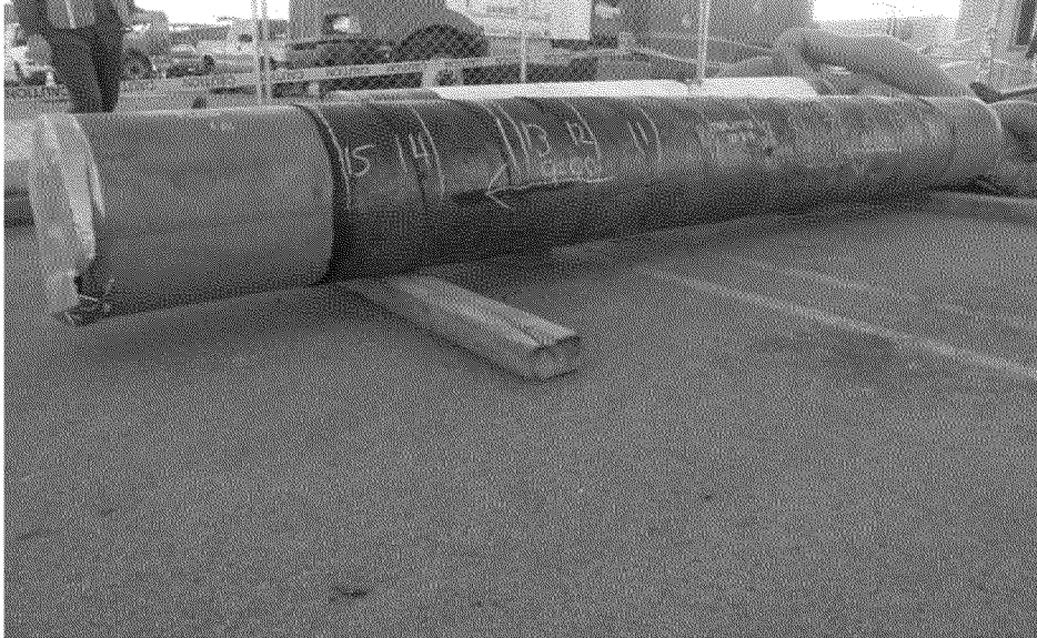
Removed pipe section coating assesment 9:00
