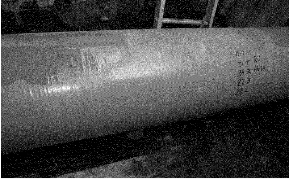
Overview of final coating condition 3:00
