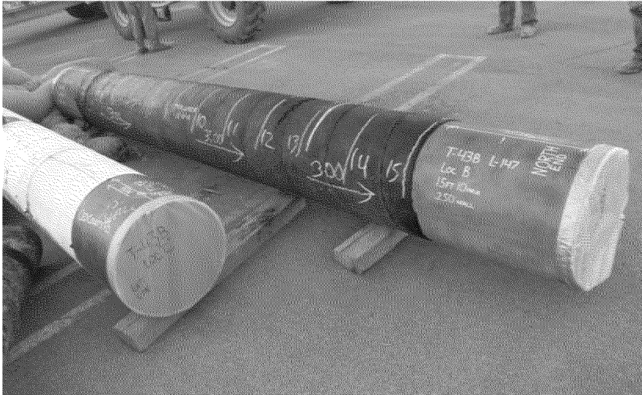
Removed pipe section coating assesment 3:00
