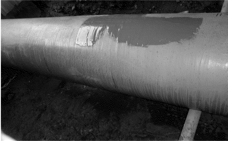
Overview of final coating condition 3:00
