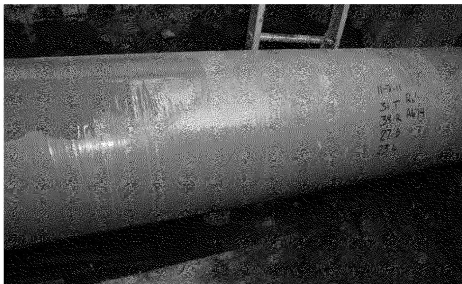
Overview of final coating condition 3:00
