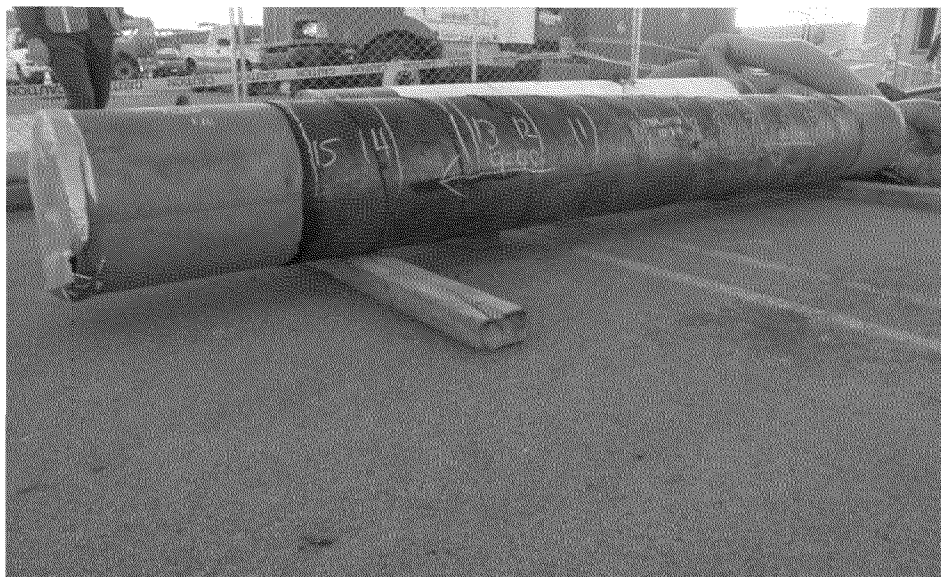
Removed pipe section coating assesment 9:00
