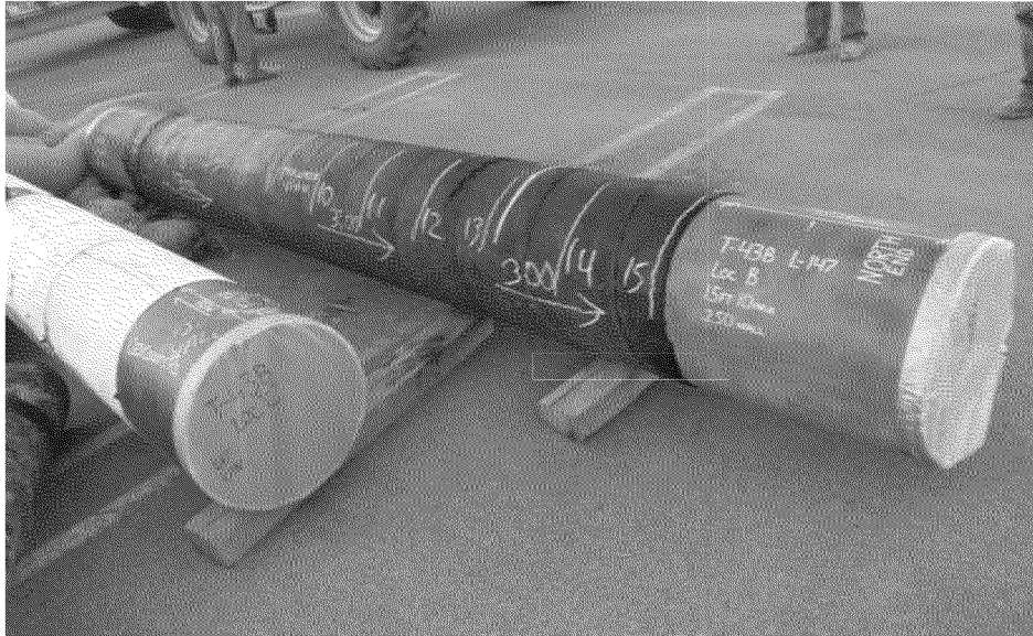
Removed pipe section coating assesment 3:00
