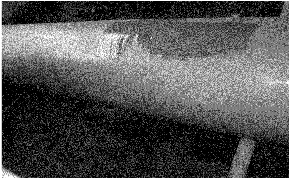
Overview of final coating condition 3:00
