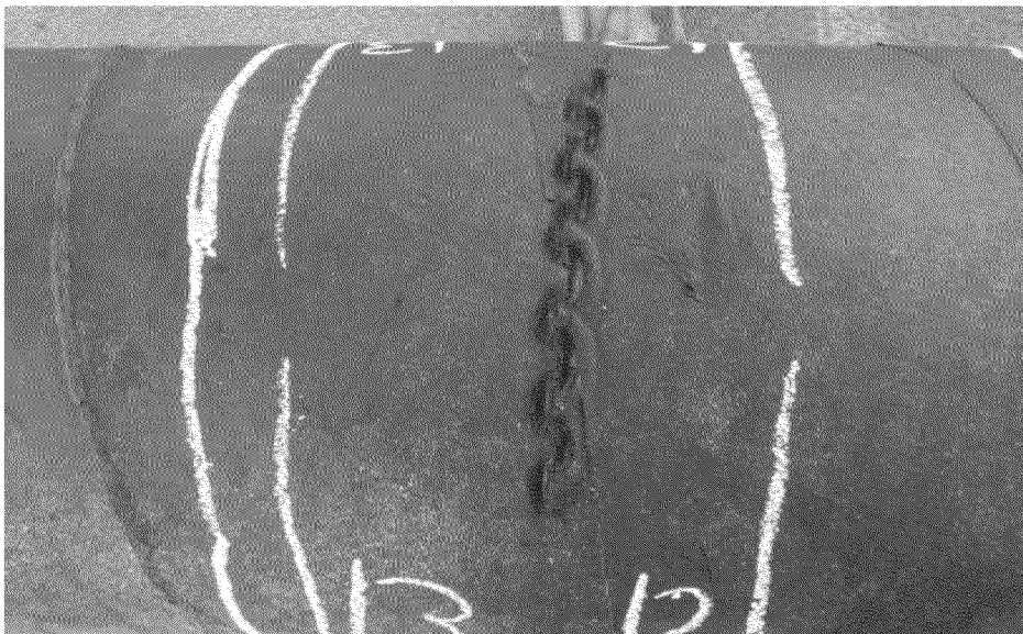
Coating damaged from removal process.
