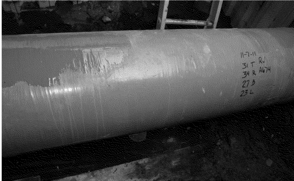
Overview of final coating condition 3:00
