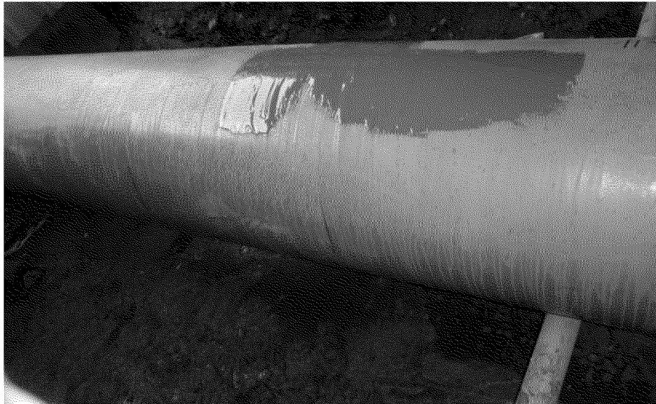
Overview of final coating condition 3:00
