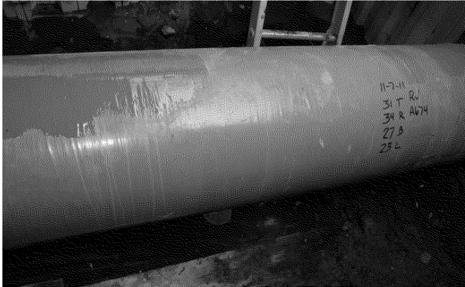
Overview of final coating condition 3:00
