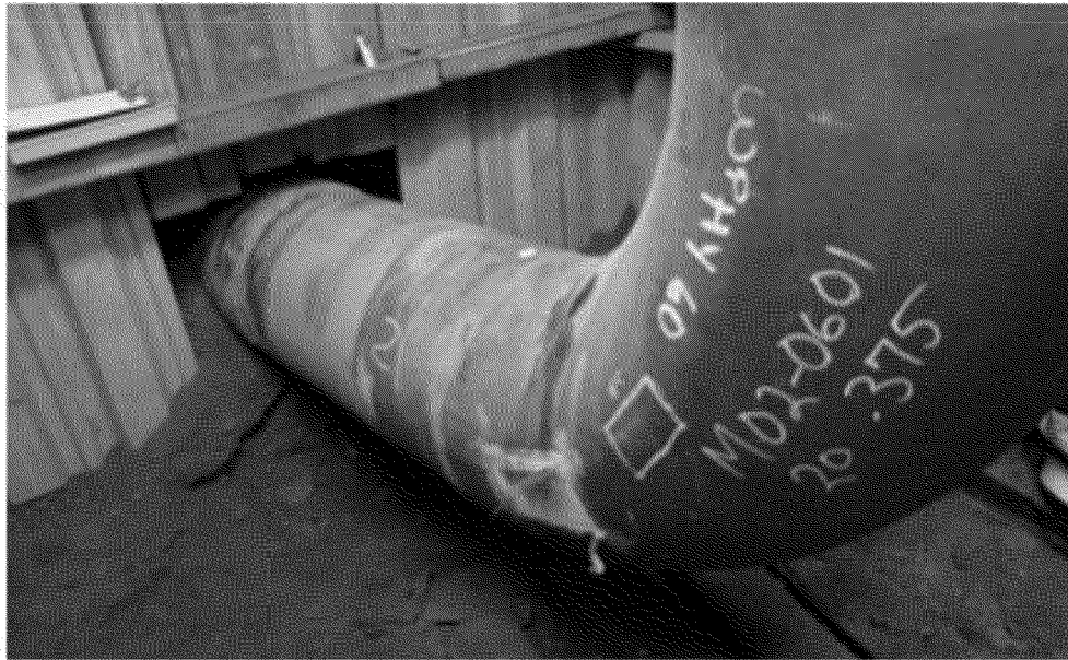
Overview of coating condition -1ft to 2ft, 3:00 position
