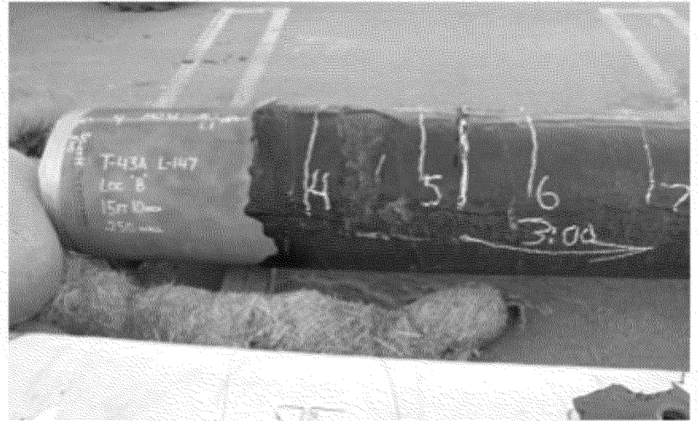
Overview of coating condition 300 position
