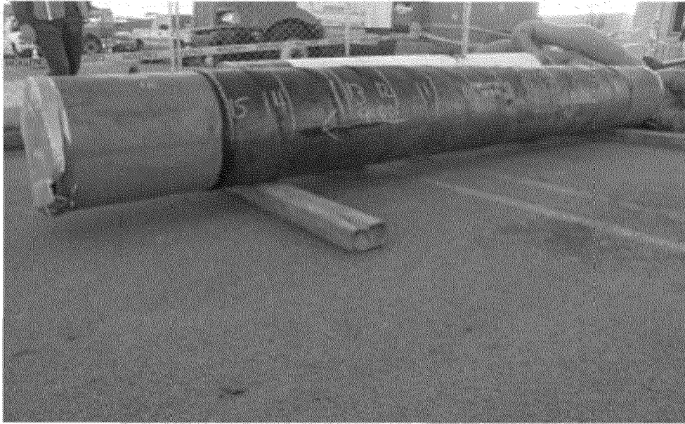
Removed pipe section coating assesment 9:00
