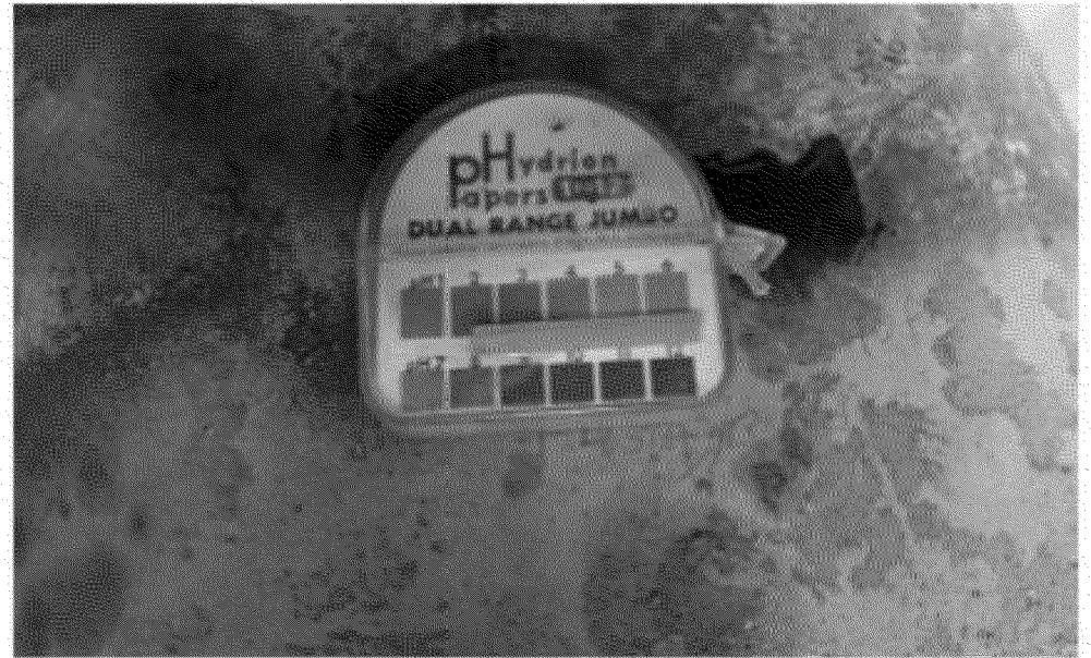
Closeup of pipe Ph.
