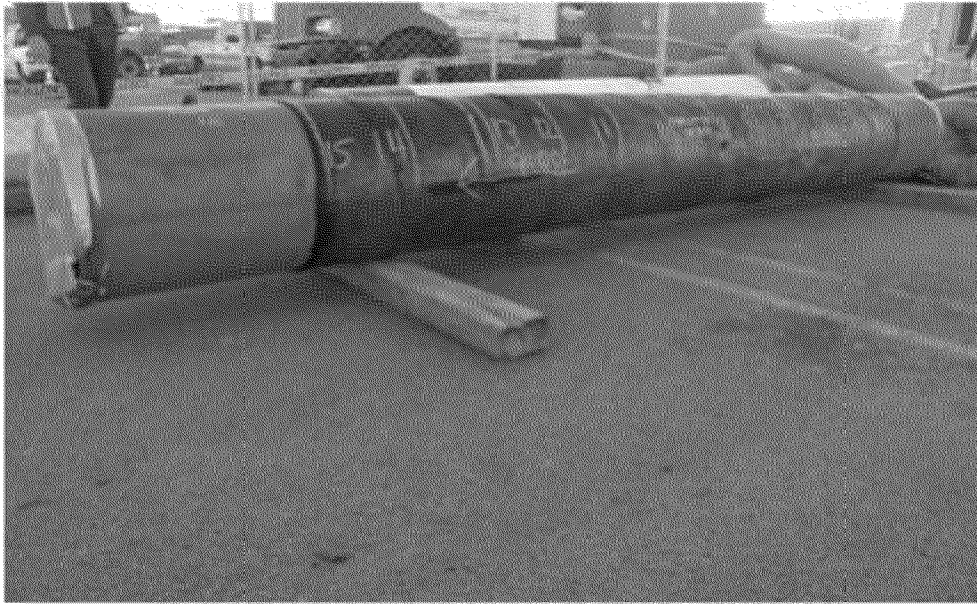
Removed pipe section coating assesment 9:00
