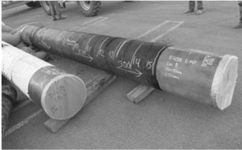
Removed pipe section coating assesment 3:00
