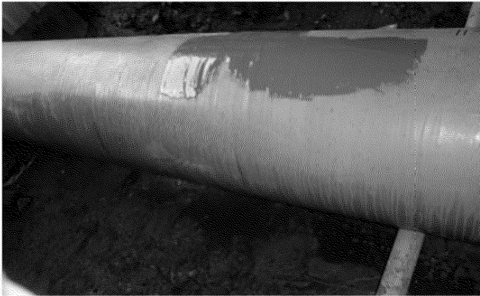
Overview of final coating condition 3:00
