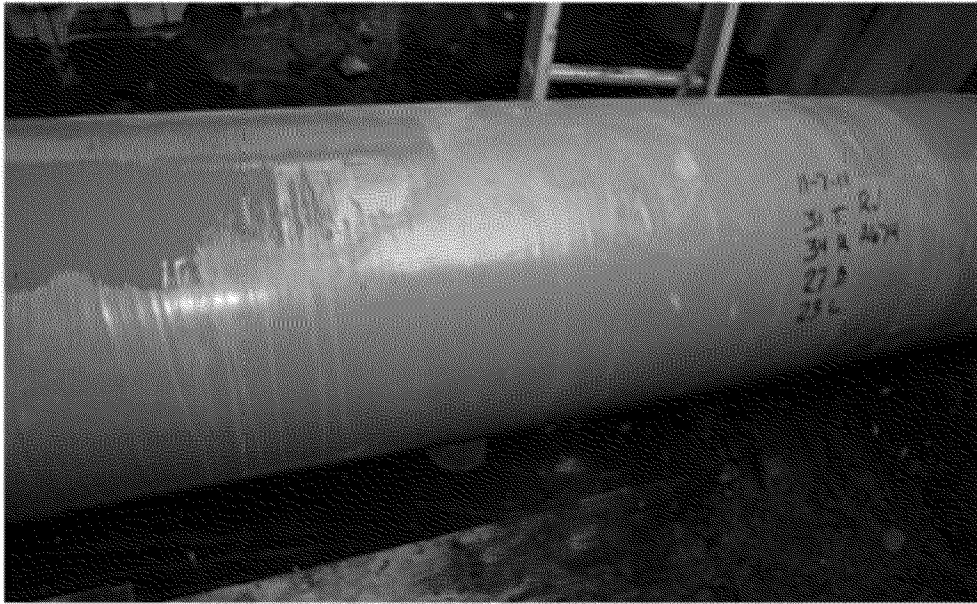
Overview of final coating condition 3:00
