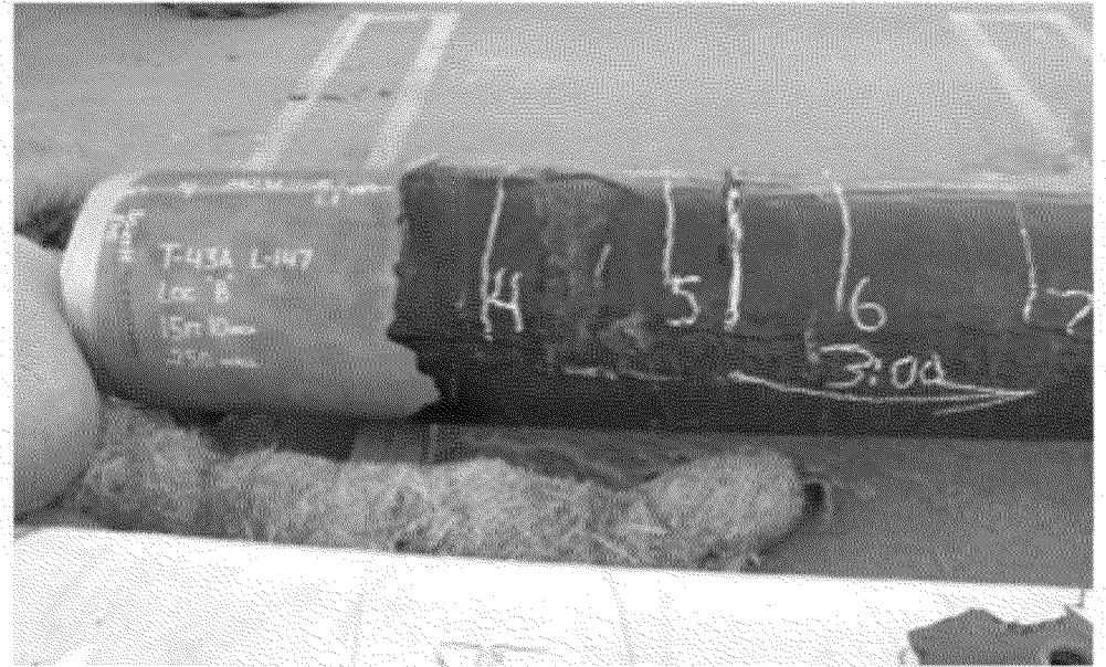
Overview of coating condition 3:00 position
