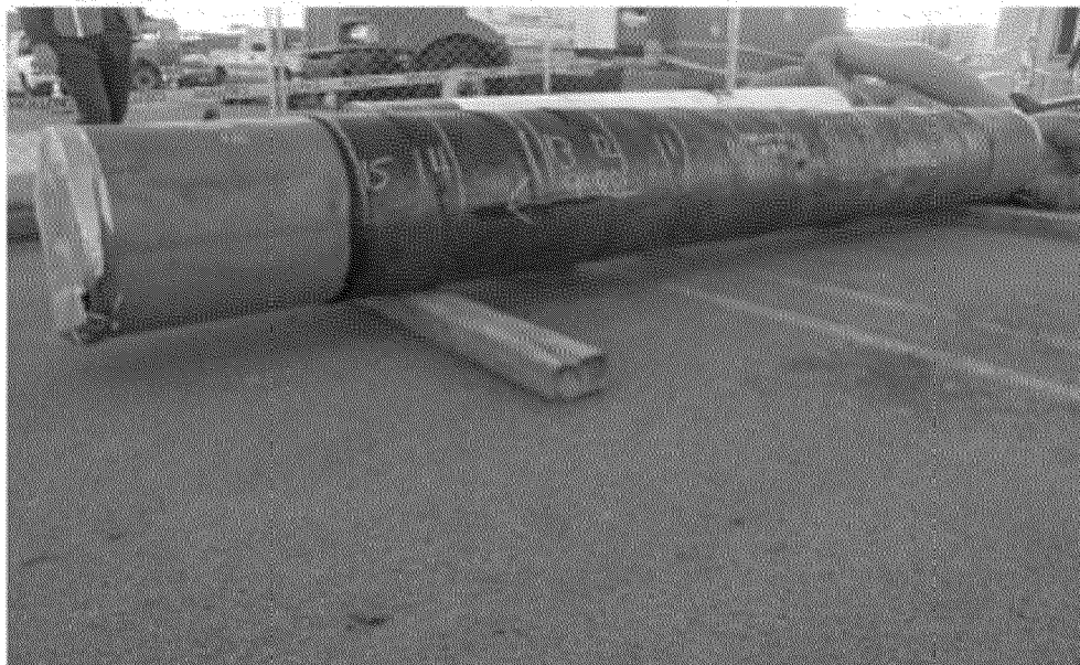
Removed pipe section coating assesment 9:00
