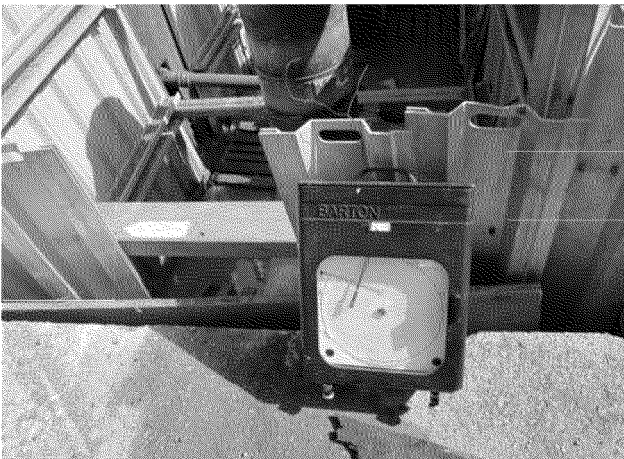
Test 42 Loc.B restrained pipe temp. recorder
