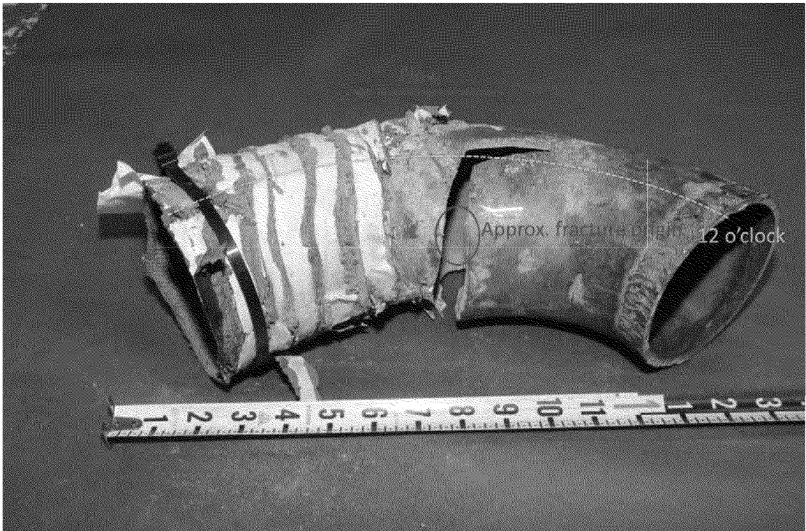
Figure 15. Image of fractured elbow.
