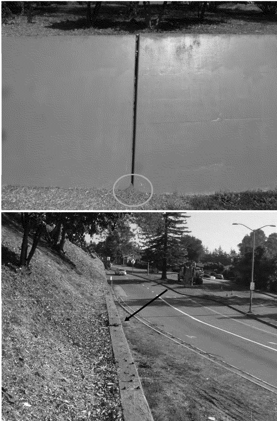
Figure 32. Displaced retaining wall joint. Oval encloses observed recent soil deposits near the base of the wall. Arrow indicates right-lateral displacement at top of wall. Photographs by Exponent, December 13, 2013.
