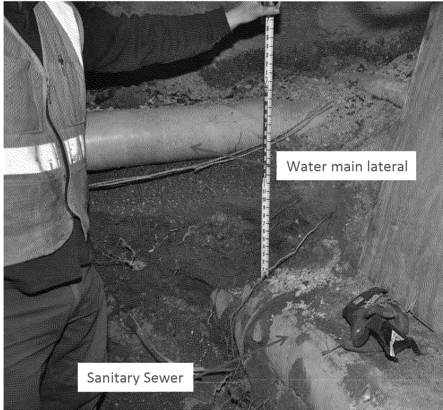
Figure 13. Water main lateral and sanitary sewer.
