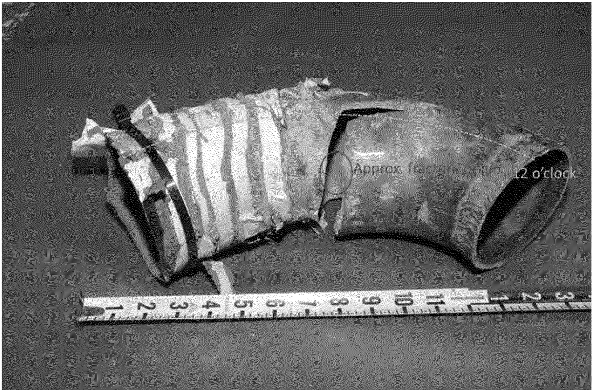
Figure 15. Image of fractured elbow.
