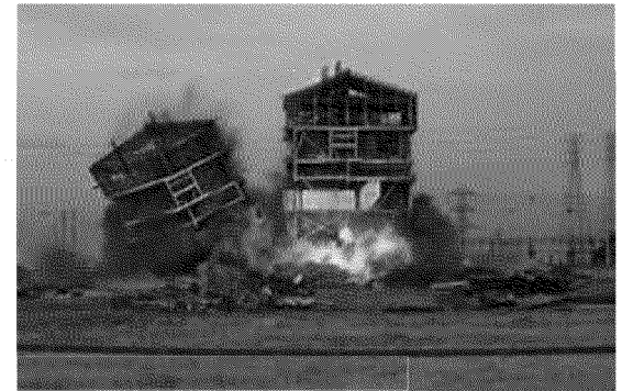
2012 & 2013 Kern Power Plant Incidents
