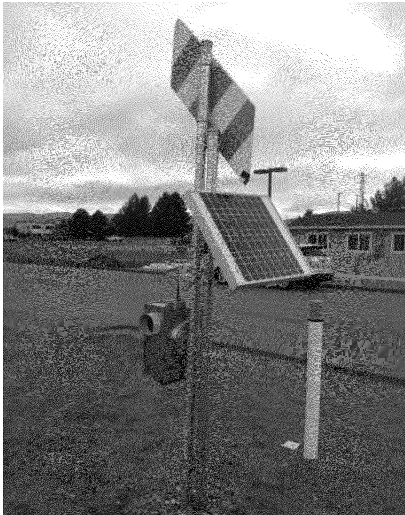
Installed Remote Methane Leak Detector at PG&E Livermore Training Center (February 2013)
